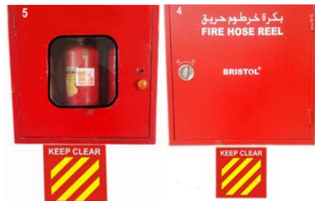
Fire Extinguishers Box
